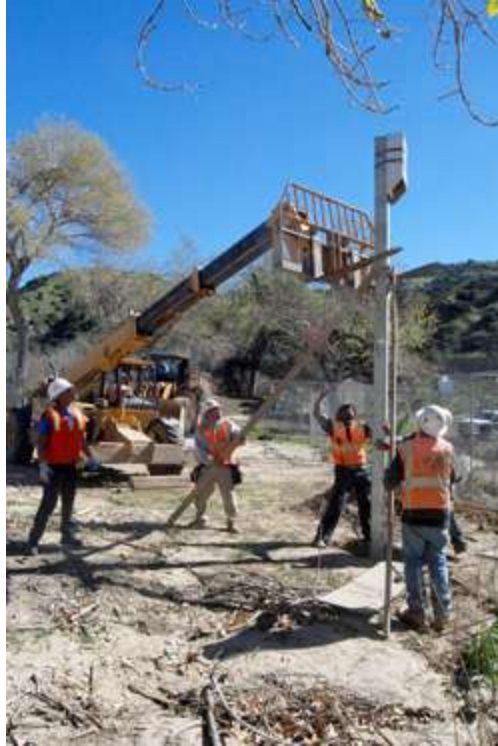
Workers adjust temporary supports designed to hold the bat box in place after the cement footing is poured. This bat box could hold up to 500 bats until construction on the new “bat friendly” bridge is completed. (USACE photo by Greg Fuderer)
